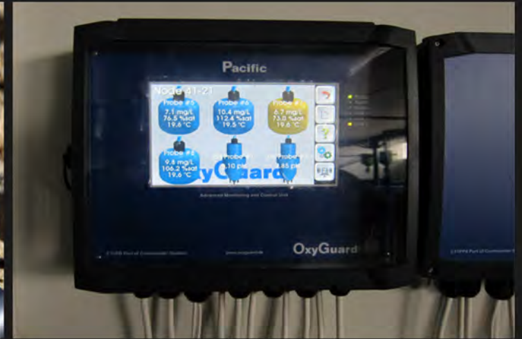
Complete monitoring and control systems
