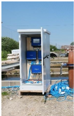
OxyGuard Pacific system on control-raceways.
