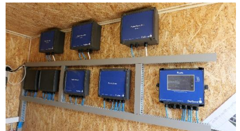
OxyGuard Pacific monitoring and control units installed within the treatment containers.
